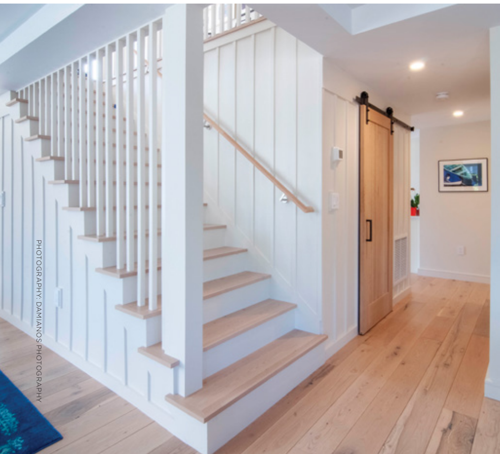
The team renovated the kitchen and installed a new staircase. One immediately takes notice of the unusual vertical balusters running the full height of the stairs. “We wanted something that wouldn’t warp,” Nino said. “I love this home.”
